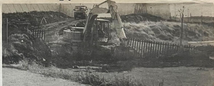
● Residents have expressed their anger that it has taken three years to commence work on a wall between Springfield Park and Springmartin
