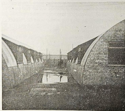
3. We live and sleep in the huts shown. The end walls are built of porous concrete brick. During heavy rain, water saturates them and flows over the hut floors. Bed clothing and wearing apparel are in a constant state of dampness. One morning the writer, an ex-internee, mopped up two full buckets of water surrounding a bed in which lay an elderly internee who was confined to bed with flu and a chest complaint.
