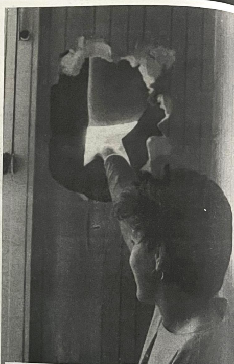
● Tracey McCabe showing damage to her mother's Divis home and (above left) two holes in the wall of the bedroom are clearly visible on either side of the bed
